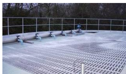
Rehabilitation of a former thickener in AQUA-RM ®
