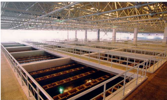
EQUIFLUX® integrated into a building
